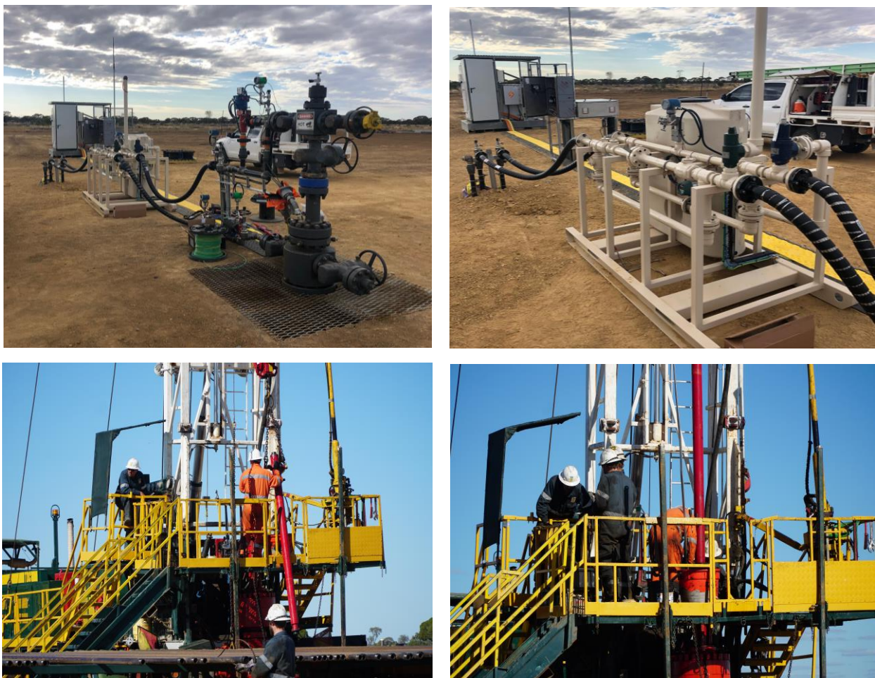
Figure 2 – Installation of surface equipment at Glenaras 14L and install of ESP on TDC Rig 8 at Glenaras 15L.
